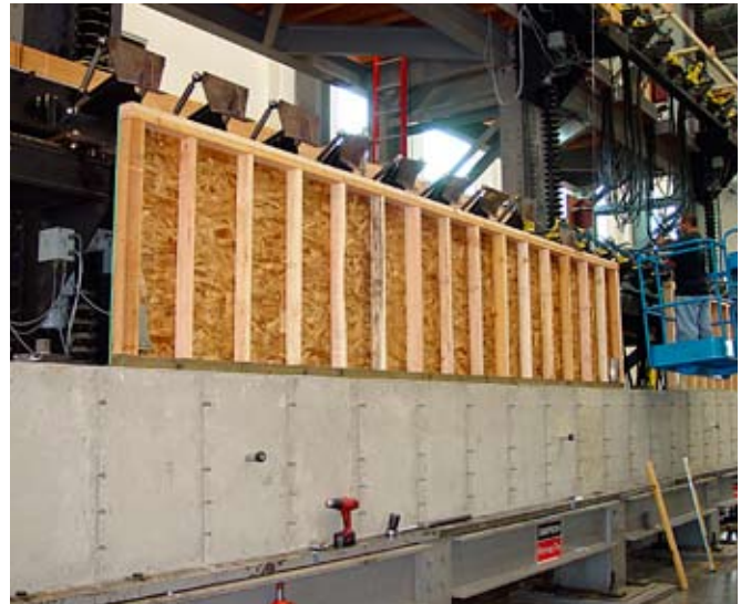
Simpson Strong-Tie performed full-scale shearwall cyclic tests using MASA mudsill anchors at the Tyrell Gilb Research Laboratory
