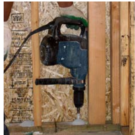
Reduces the need to retrofit anchors to account for misplaced anchor bolts
