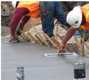
Eliminating anchor bolts makes finishing easier and results in a flatter slab
