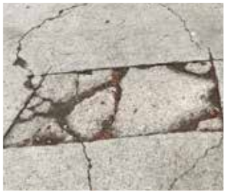
Cracked and spalled concrete.
