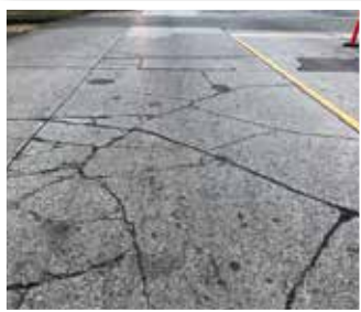
Distressed concrete road in high traffic industrial area.
