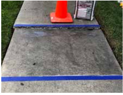
A trip and fall liability hazard.
