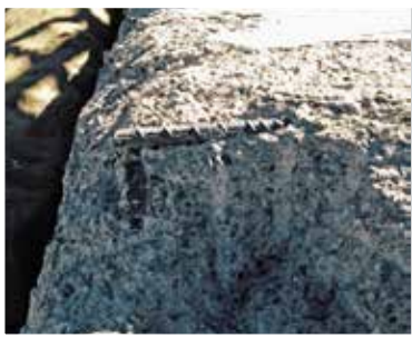
Spalled concrete with exposed rebar.
