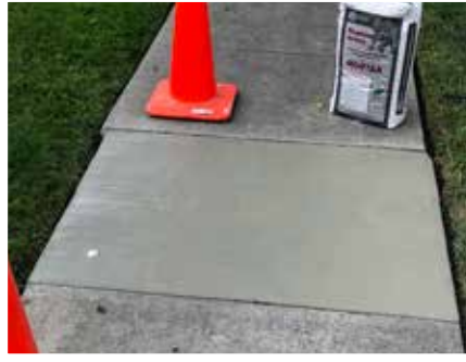
The area was resurfaced with Elephant Armor® without deconstructing the failed surface.
