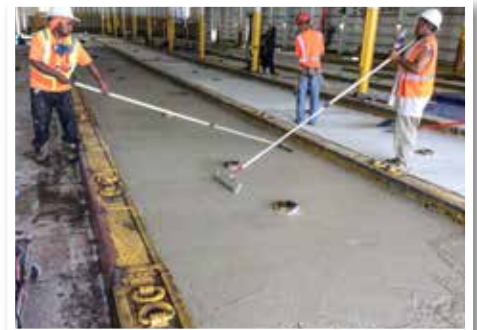
This permanent repair can be done at a fraction of the cost and at a significantly reduced time frame.
