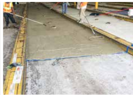
Elephant Armor® overlay is rolled and finished over existing primed concrete to a thickness of 1/2".
