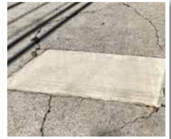
Spall repair one year after placement.
