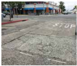
Failing broken and degraded concrete panel.
