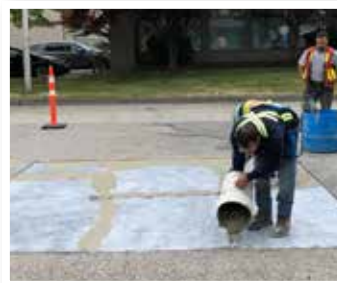
The area is primed with Elephant Armor® Primer and large cracks filled with Elephant Armor®.
