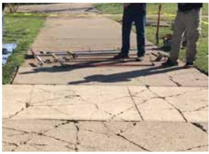
A severely cracked and degraded sidewalk.
