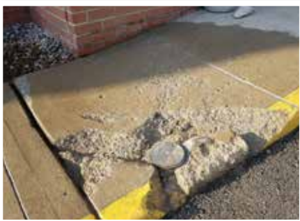
Severely degraded sidewalk causing trip hazard.
